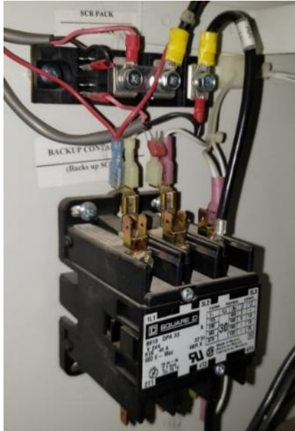
Figura 42. Contactor de Backup.
