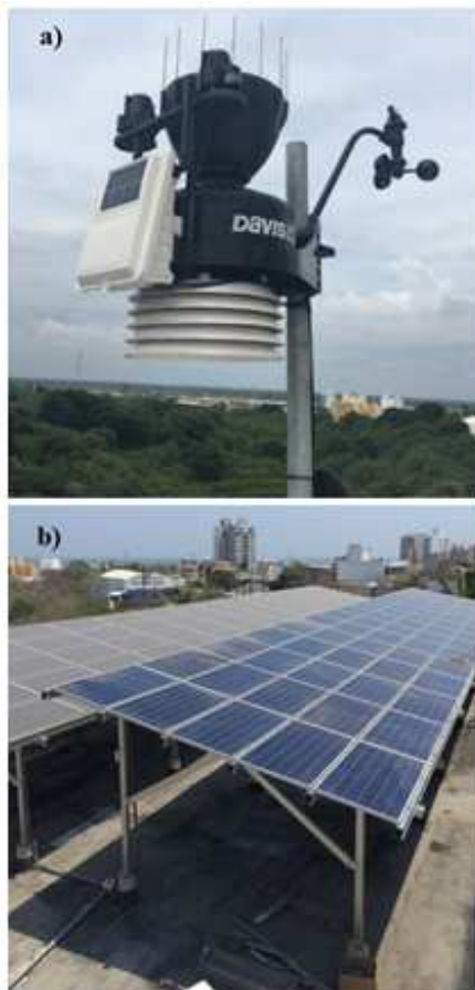
Fig. 1 Experimental setup, a) Meteorological station, b) Solar generation plant
